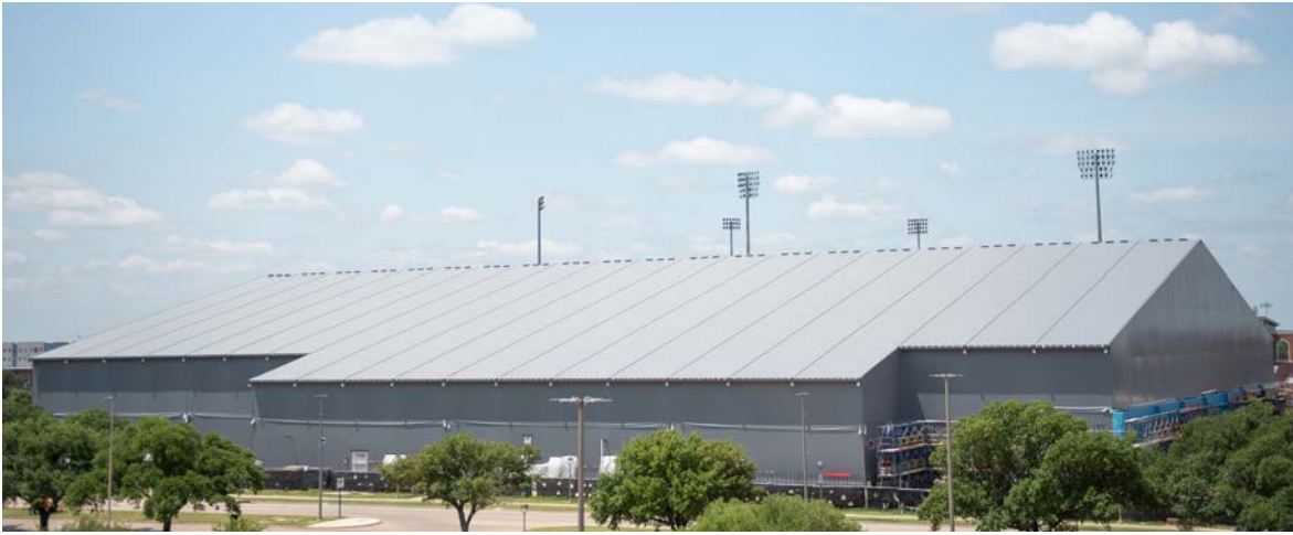
The new R.A. "Murray" Fasken '38 Indoor Track construction is slated to be completed in the fall of 2023 with Aggie Track & Field prepared to host indoor competition in the facility next season.
